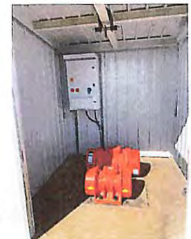
One of four sets of SOVs installed near the RTE plant.
